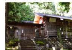
27 Hakusan Shrine (Okuwa Village) C-5 Built in 1334, it is the oldest remaining shrine building in Nagano.
